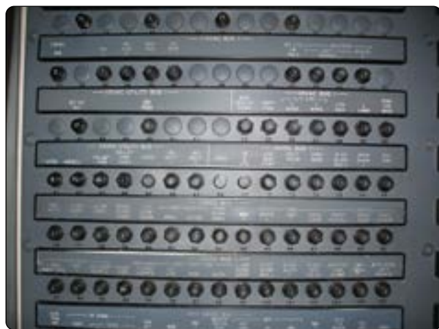
Figure 9-173. Circuit breaker panel.
