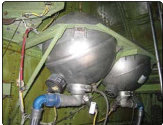
Figure 17-12. Built-in non-portable fire extinguisher containers (HRD bottles) on an airliner.
