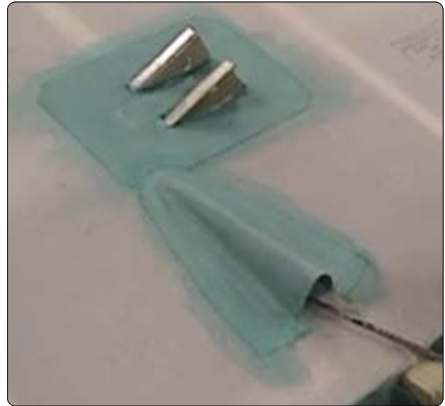
Figure 3-33. A strut fitting and cable guide with reinforcing fabric gussets cemented in place.
