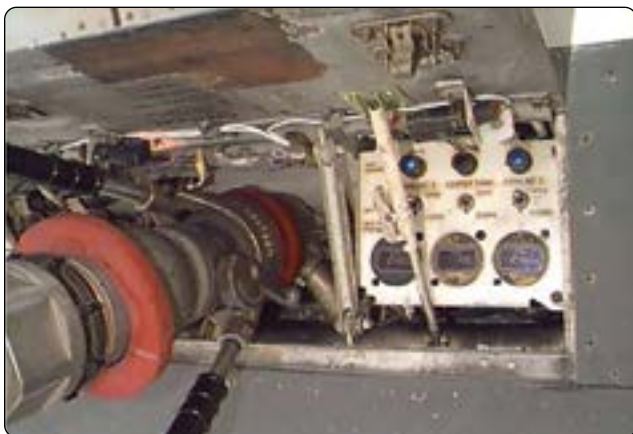
Figure 14-21. A central pressure refueling station on a transport category aircraft allows all fuel tanks to be filled from one position.
