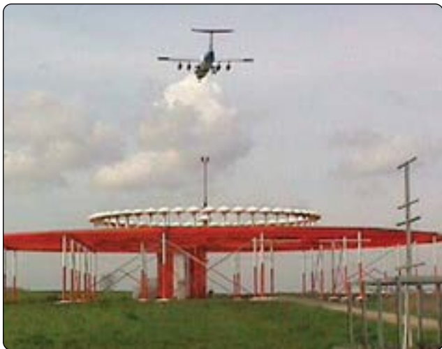
Figure 11-119. A VOR with DME ground station.
