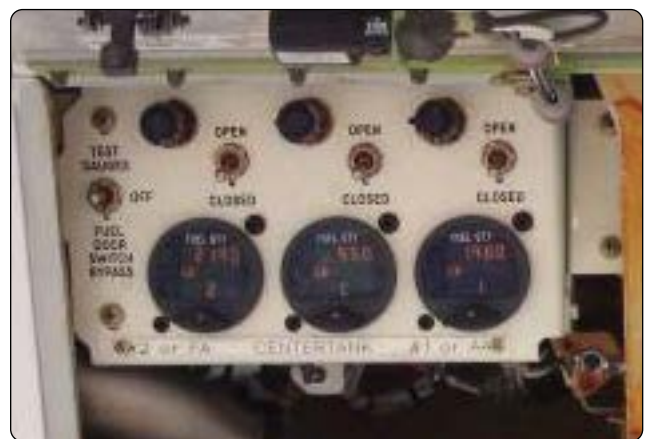
Figure 14-106. This panel at the pressure refueling station has valve position switches and quantity gauges to be used during refueling. Valve open position lights are adjacent to the switches for each tank.
