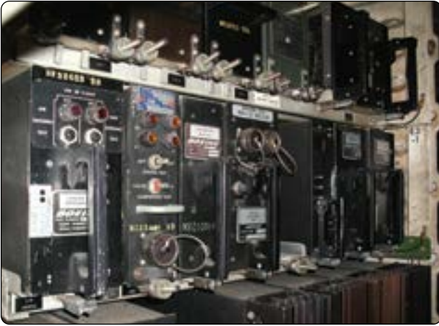
Figure 9-81. Line replaceable units in an equipment rack.
