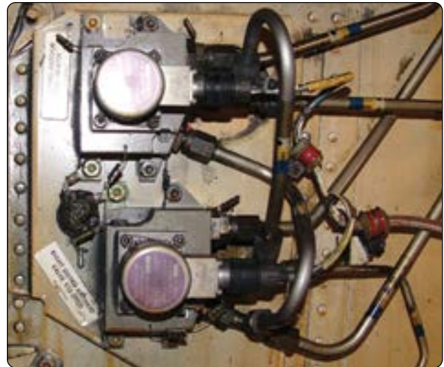
Figure 13-112. Two anti-skid control valves with associated plumbing and wiring.
