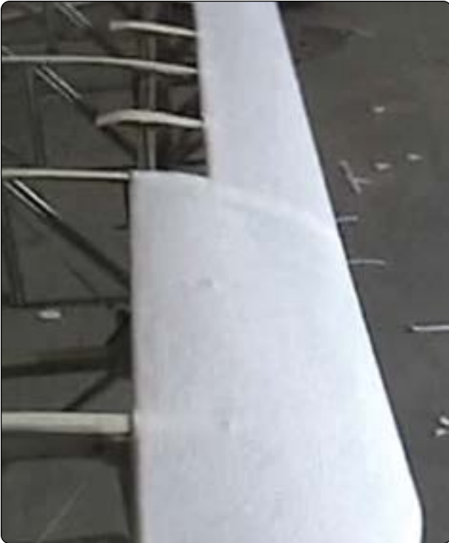
Figure 3-17. The use of specified felt or padding over the wing leading edges before the fabric is installed results in a smooth regular surface.
