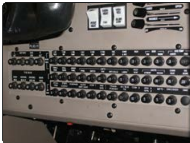
Figure 9-83. Light aircraft circuit breaker panel.
